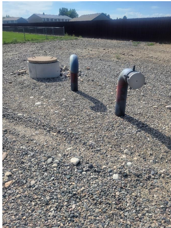
Existing Dry Hydrant
