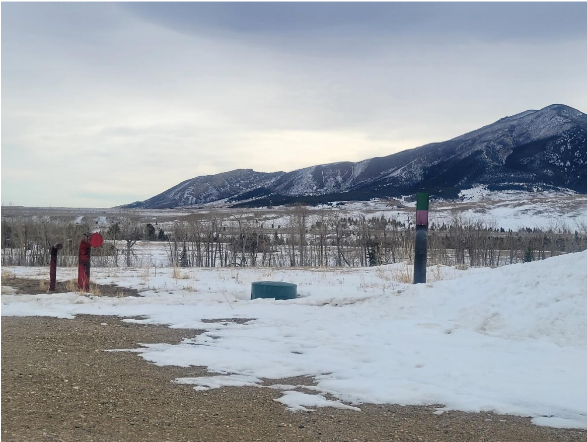
Existing Dry Hydrant
